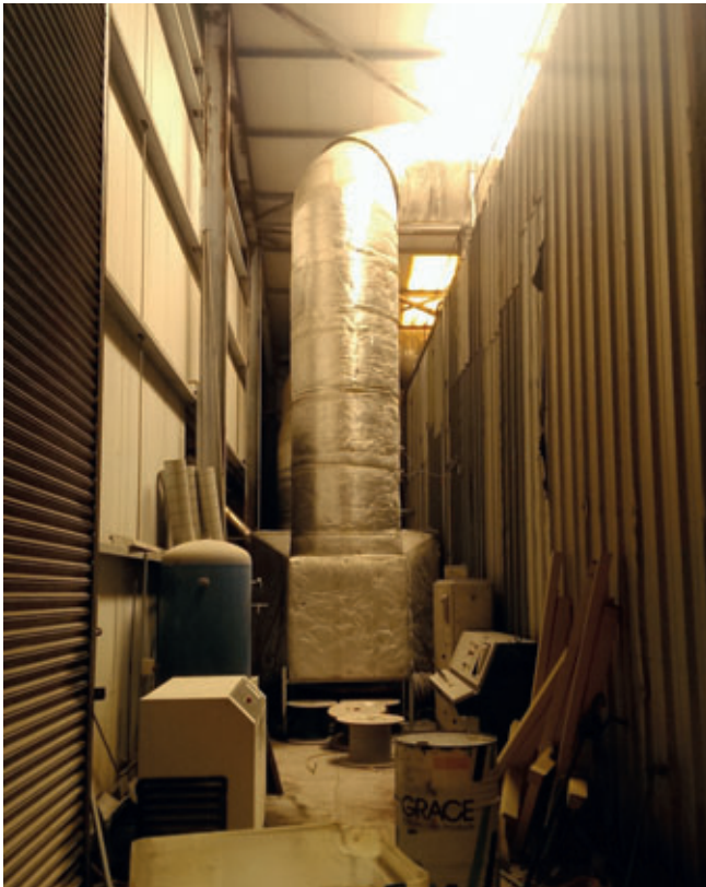
Before: oversized air heating unit, "insulated" with foil coated fibreglass wool and mounted with chicken wire. Insulation panels on chamber were leaking and joints (connection between walls and ceiling panels) were not sealed.
