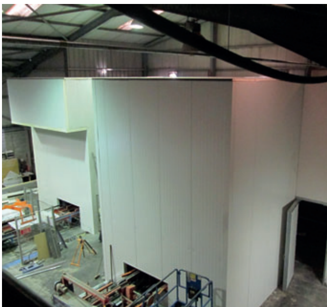
After: elevator & lowerator enclosed with insulation panels during construction. Space for raised maintenance platforms and equipment door for access
