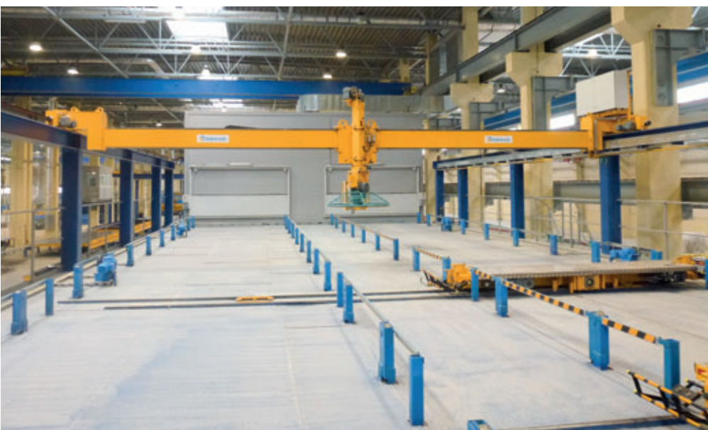
Following the pre-curing of the concrete in the pre-curing chamber the pallets are moved by the lifting transfer table to the 2nd level. A power trowel and four smoothing stations are available there for the fine smoothing.
