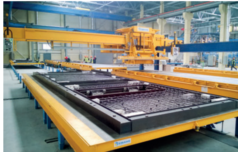
The finished shuttered pallet is ready for concreting. The concrete is discharged evenly by a screw system in accordance with the data sent by ebos. The concrete layer is drawn off and smoothed to the desired height by a vibrating levelling beam.
