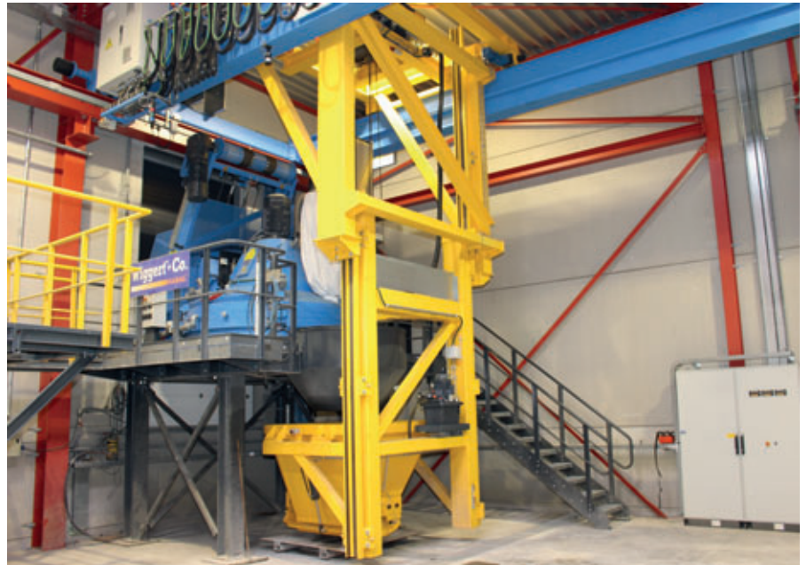
The batching plant contains an Ebawe special concrete distributor as well as a Wiggert planetary mixer
