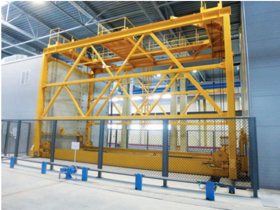
The pallets are placed into and removed from the curing rack by the lifting transfer table.
