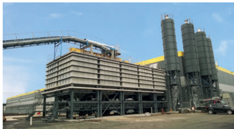
Zapad also invested into a completely new mixing plant, which supplies the required fresh concrete for the complete product range.
