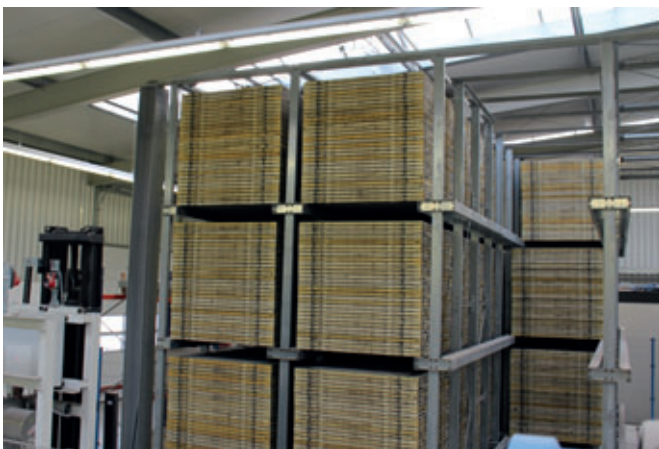
Board buffer rack for 2,800 underlay boards
