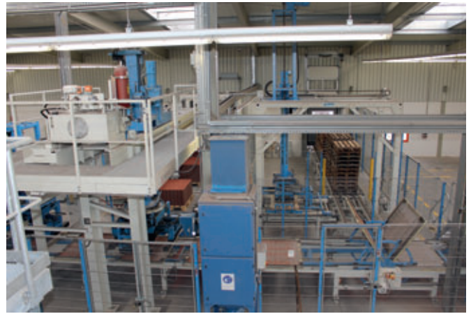
The empty underlay boards are cleaned, turned and stacked, after which the finger car either places them in the board buffer rack or takes them to the concrete block making machine.
