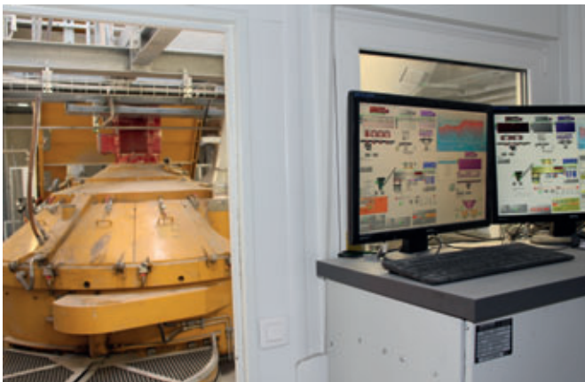
All mixing and dosing processes are controlled by the Sauter controller.
