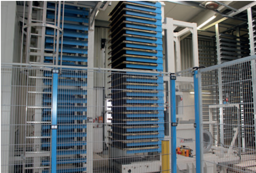
The elevator can accept 23 underlay boards, which are then taken over by the Hess finger car and driven into the rack system from Rotho.
