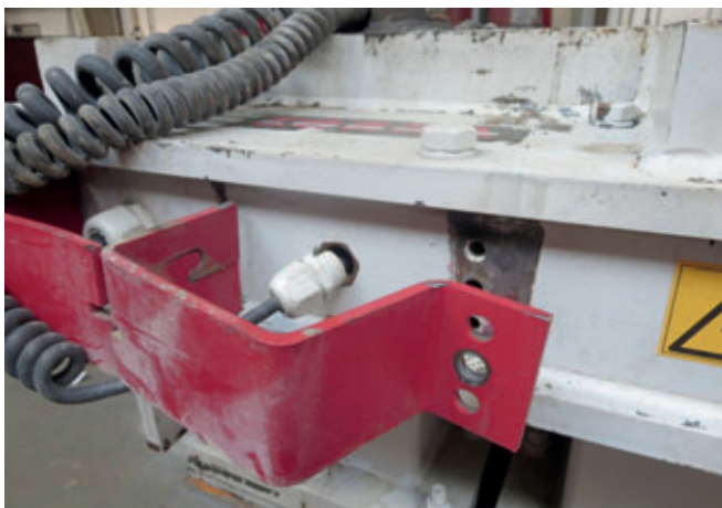
Damage due to incorrect handling / maintenance
