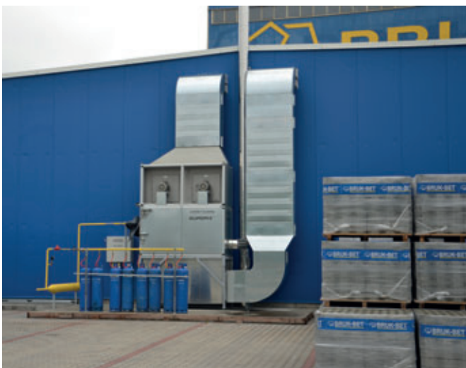
Quadrix AHU Heating and Circulation Unit shown outside of the curing chamber prior to the construction of the equipment shed
