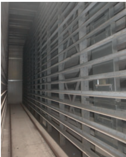
Picture taken during curing with a temperature equal to 35°C (100°F) and a relative humidity of 100% - dry floor, rails and racks. The air supply duct with louvers located to the right of the picture.
