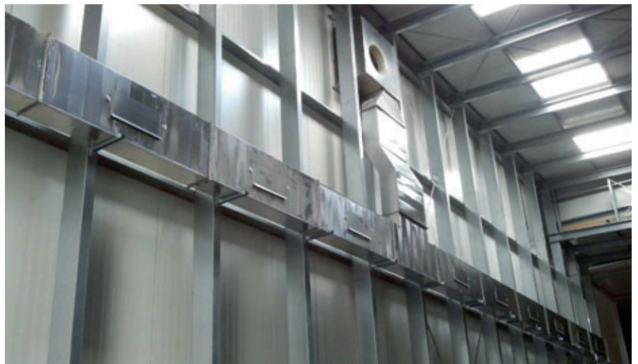
Picture of transfer car area taken with chamber temperature of 35°C (100°F) and relative humidity of 90%. The floor and walls are very dry and there is not any fog or haze which is important for the operation of transfer cars using laser positioning.
