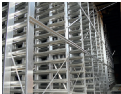
The curing chamber installed by HS Anlagentechnik has 22 levels with a distance between levels of 330 mm.
