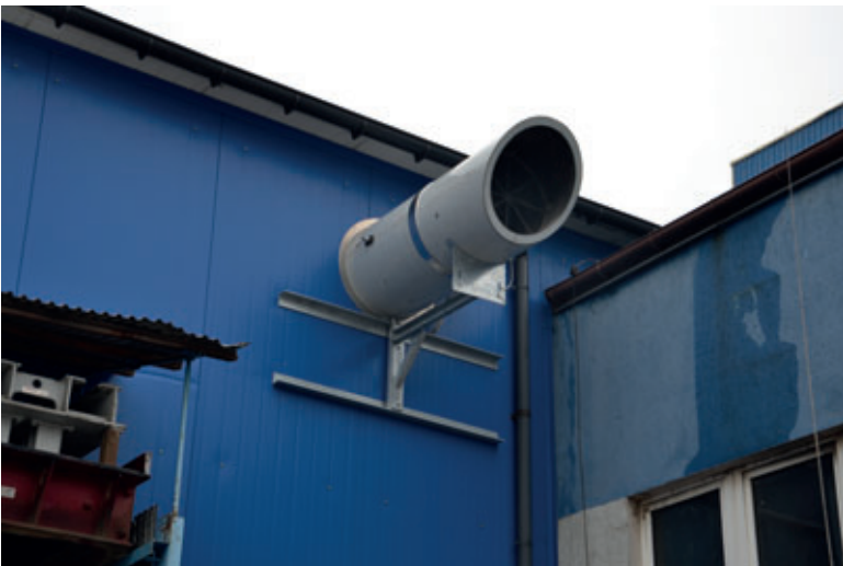
Exhaust Unit which is automatically opened and closed depending on the relative humidity of the curing atmosphere in the curing chamber.
