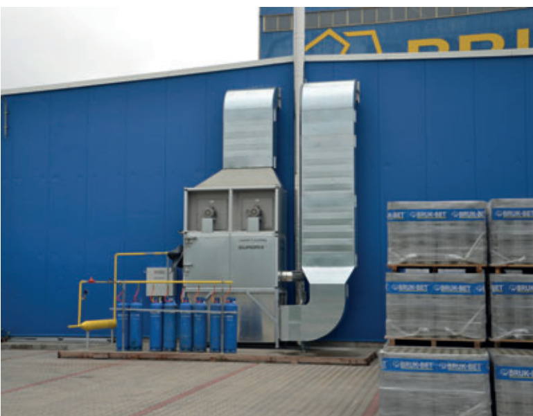
Quadrix AHU Heating and Circulation Unit shown outside of the curing chamber prior to the construction of the equipment shed
