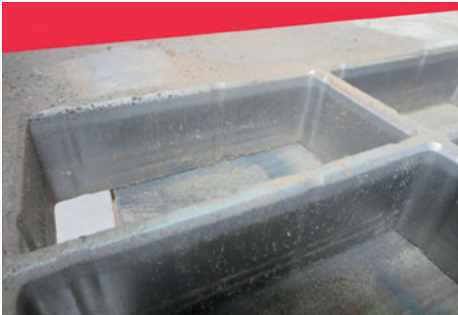
Wear in the compaction area
