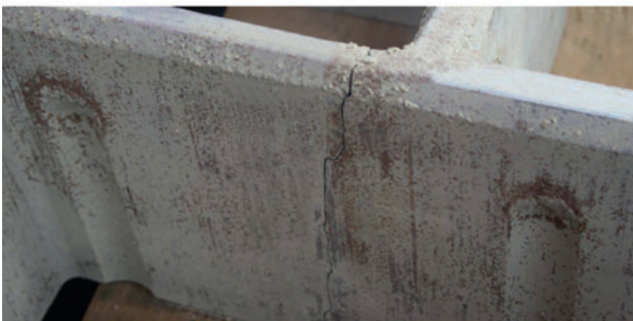
Sollicitation excessive / fissures
