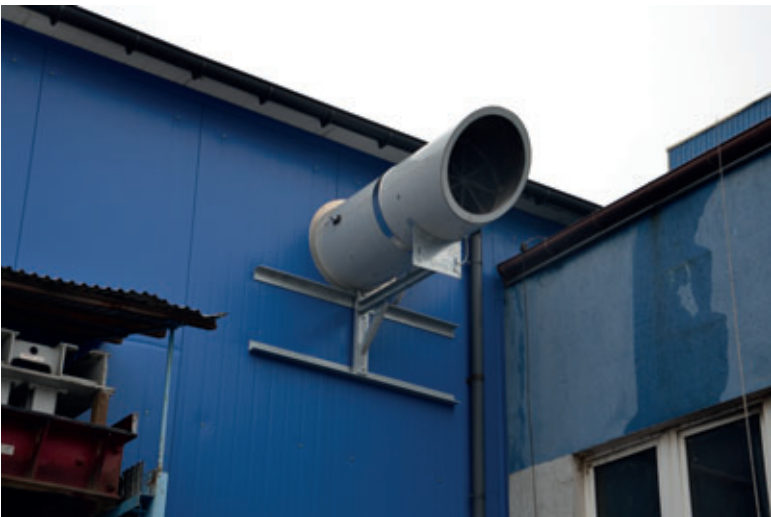
Exhaust Unit which is automatically opened and closed depending on the relative humidity of the curing atmosphere in the curing chamber.
