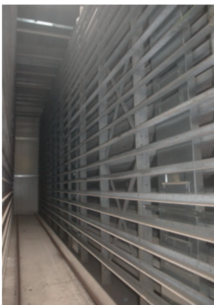
Picture taken during curing with a temperature equal to 35°C (100°F) and a relative humidity of 100% - dry floor, rails and racks. The air supply duct with louvers located to the right of the picture.
