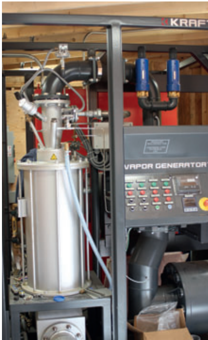
A single Kraft Vapor Generator (pictured during installation) supplies all curing enclosures of the Unistress production site with the optimal curing climate.
