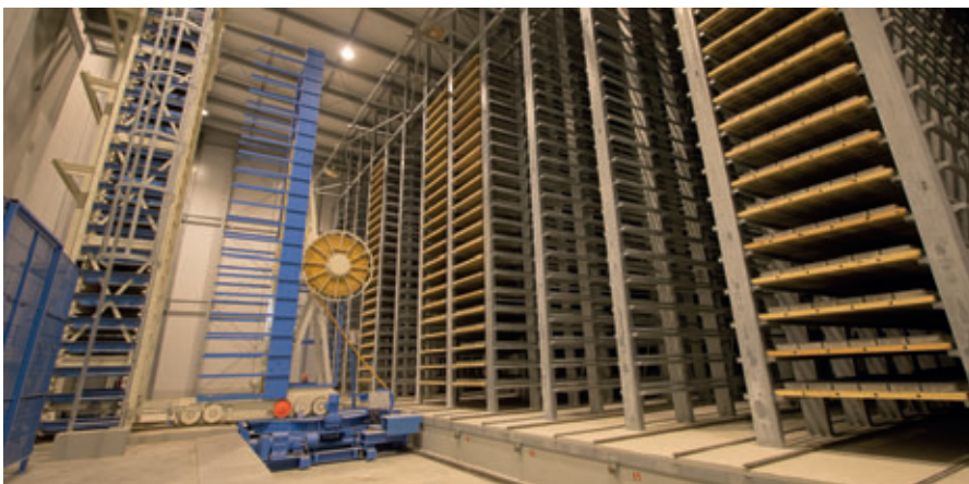
Drying chamber with racks from Rotho in the new Vibor-S plant in Russia: total capacity 8000 boards
