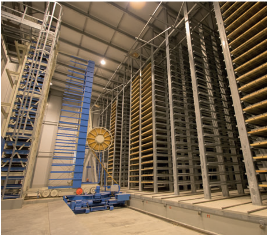
Drying chamber with racks from Rotho in the new Vibor-S plant in Russia: total capacity 8000 boards
