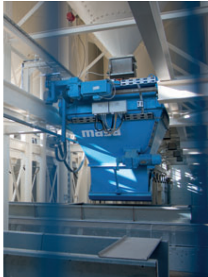
20 aggregate silos are available for filling the two charging scales
