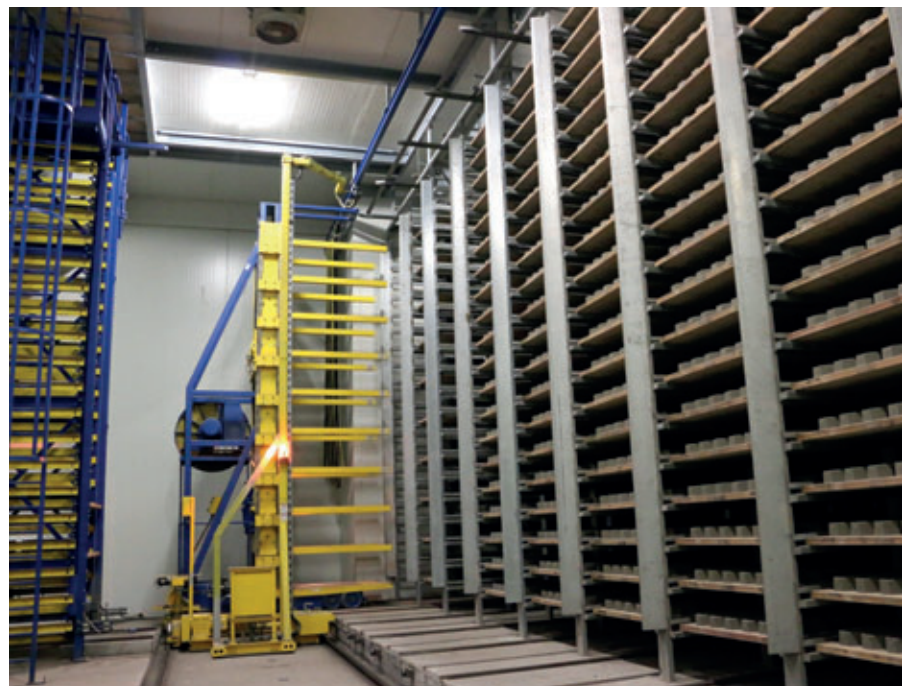
Masa transfer table with new large chamber system and ventilation system
