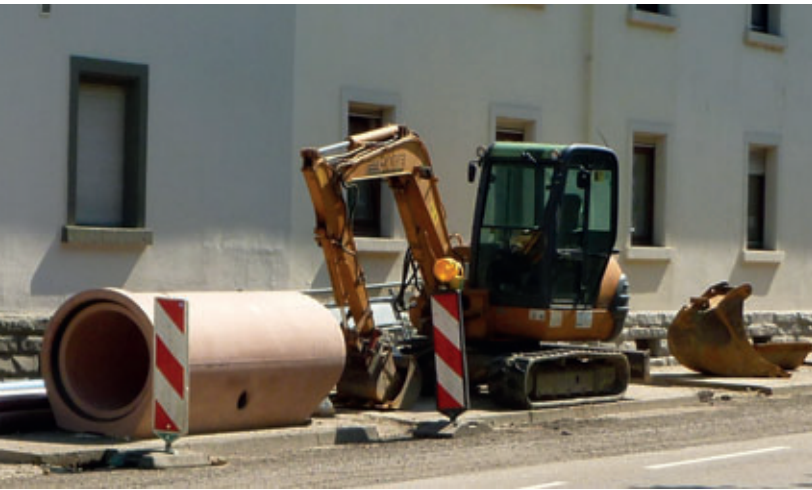
As a basis for an adjacent redevelopment, DN800 prebed concrete pipes were produced in Achern, Baden-Württemberg, some with pre-made connections for side branches on the same invert
