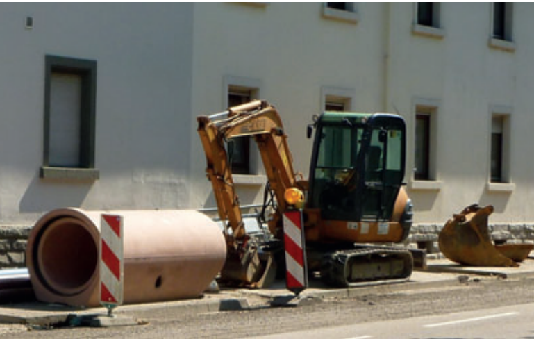
As a basis for an adjacent redevelopment, DN800 prebed concrete pipes were produced in Achern, Baden-Württemberg, some with pre-made connections for side branches on the same invert
