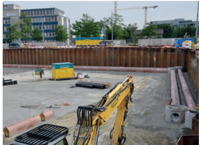
The progress of construction work – laying, filling, compacting – was significantly increased through the use of Perfect Pipe with connector in this major construction site in Zurich as described
