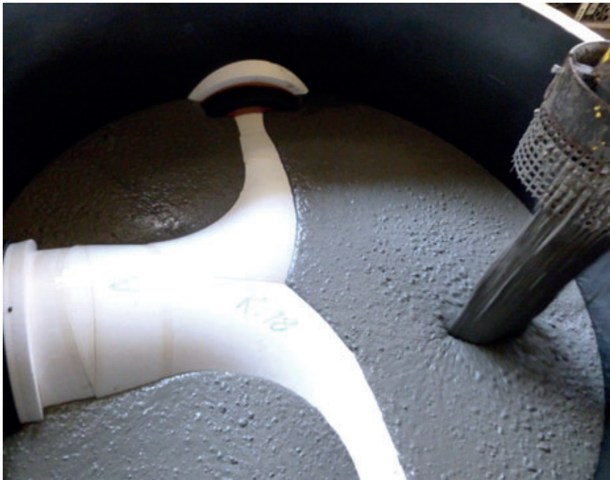
Concreting of Perfect manhole bases in steel moulds – manufacture of wet-cast components “in one pour”
