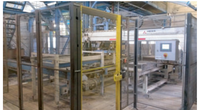
Integration of a board buffer in the existing plant
