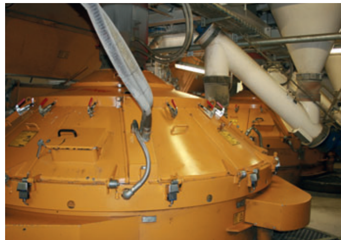
Two identical mixers from Haarup (3,750 l) were installed in the mixing tower.
