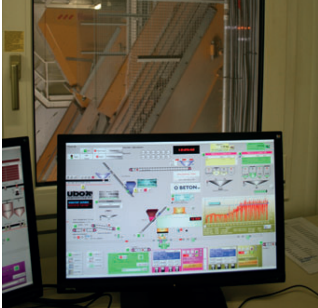
All mixing and dosing processes are controlled by the Sauter controller
