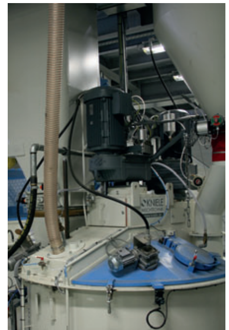
The facing concrete mixer from Kniele
