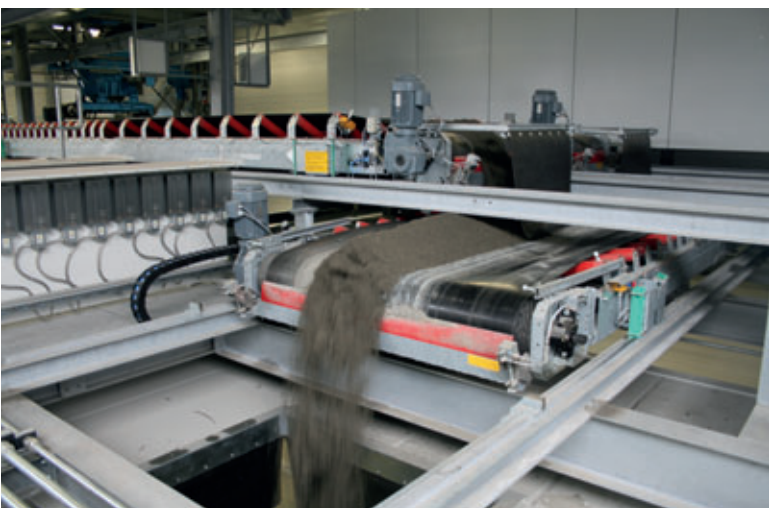
The belt conveyors from VHV Anlagenbau transport the concrete from the mixers to the concrete block making machine
