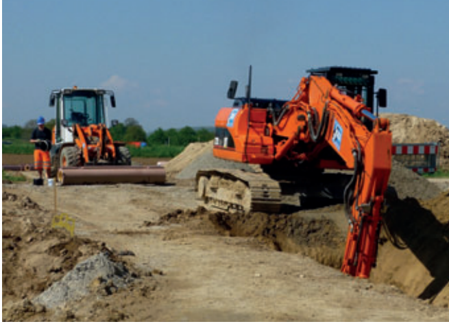
Engineers and contractors are delighted with the installation process, while end-customers are delighted with the progress and the durability of the system.
