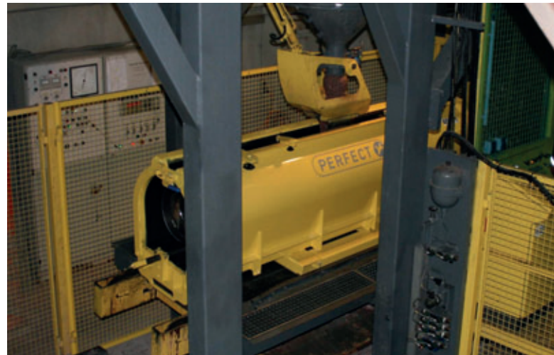
A mould sits on a movable table during the concrete pouring process.
