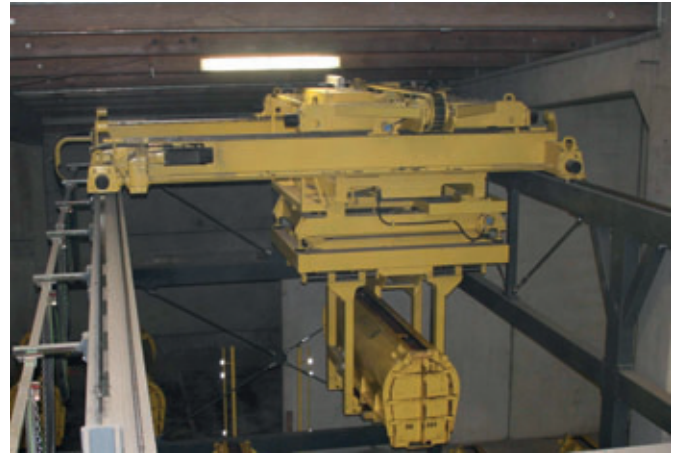
The crane takes a freshly filled mould and places it on the curing area's moving floor system.
