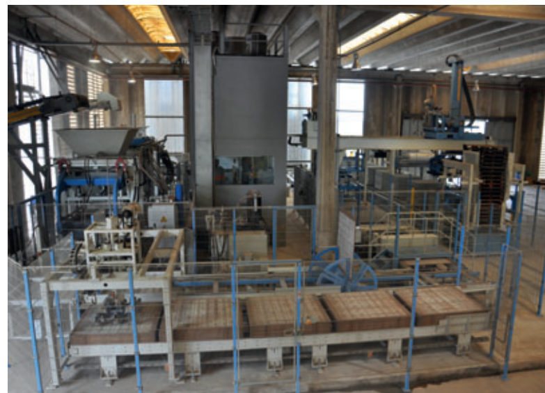
New block-making plant from the Hess Group
