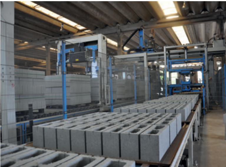
Walking beam conveyor on the dry side
