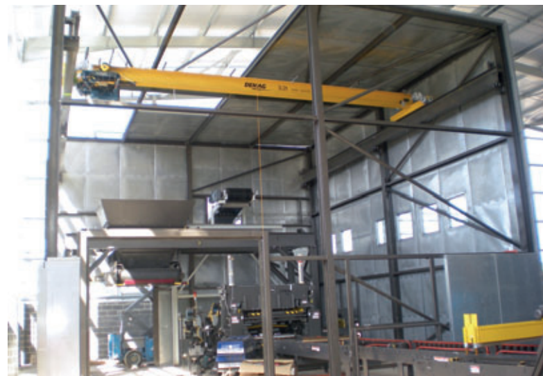
The internal structure of the acoustic booth completed with overhead crane for maintenance and mould changes
