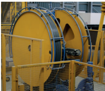
The steel wire required for pre-stressing is also brought to the plant in coils where it is processed with a wrapping speed of up to 6 m/s.
