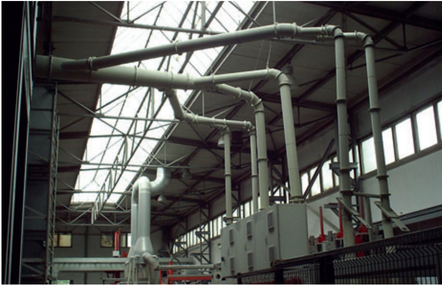
Piping to separately located suction plants
