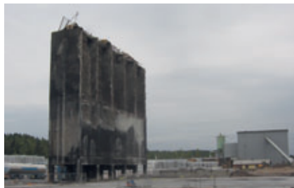
After the fire the plant was completely destroyed. Only the concrete silos could be preserved.
