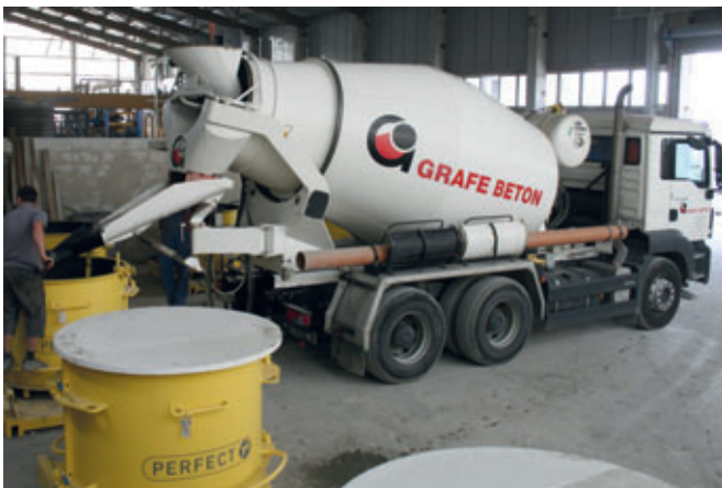
A truck mixer from Grafe's own fleet transports concrete to the production site
