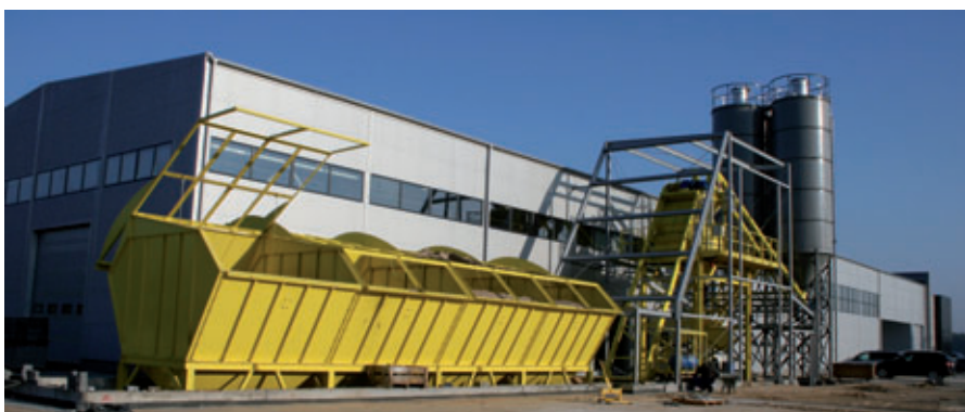
The new hall which hosts the Perfect production system at Ritbet. Insulation works at the mixing and batching plant were still in progress right after the production start.
