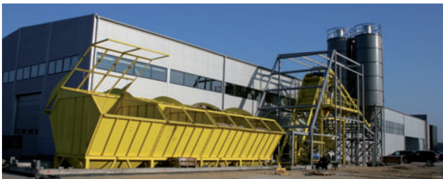
The new hall which hosts the Perfect production system at Ritbet. Insulation works at the mixing and batching plant were still in progress right after the production start.
