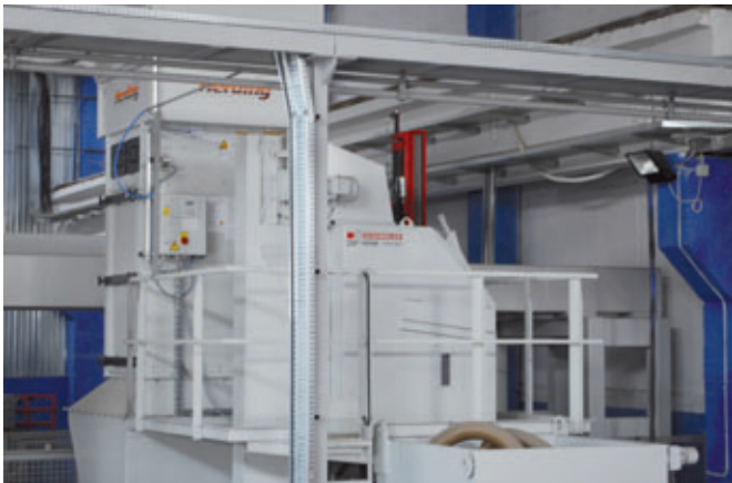
Blasting plant with sintered lamella filter
