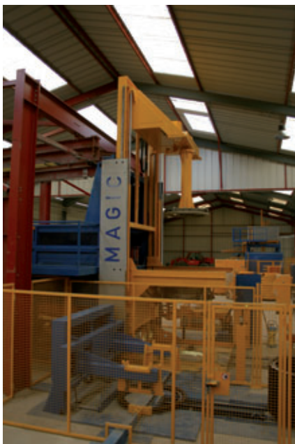
The new Magic 1501 production system at Bonna Sabla in the precast plant in Bruz
