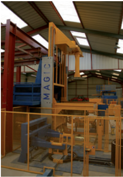
The new Magic 1501 production system at Bonna Sabla in the precast plant in Bruz
