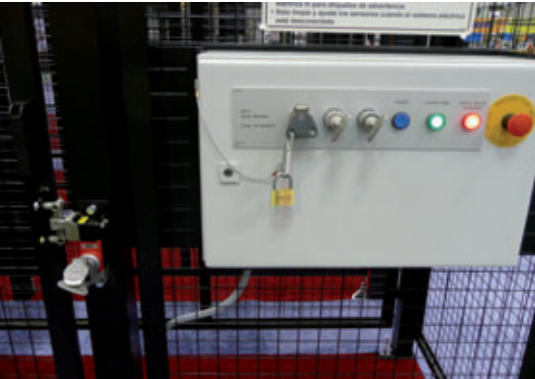
Securing method using a personal padlock
