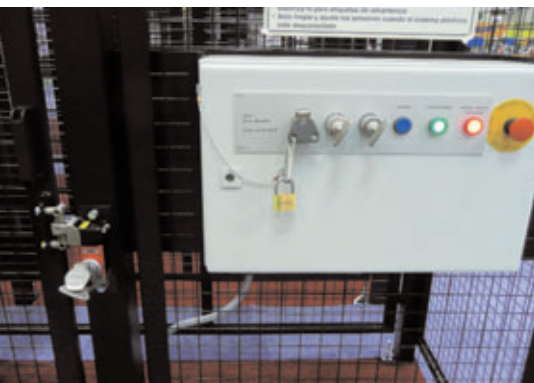
Securing method using a personal padlock
