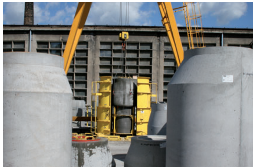
After sufficient hardening time, the moulds are opened again and the manhole cones are carefully lifted by crane out of the mould
