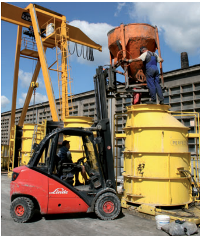
Concreting is done with a forklift and concrete bucket; as with the Perfect System, only self-compacting concrete is used
