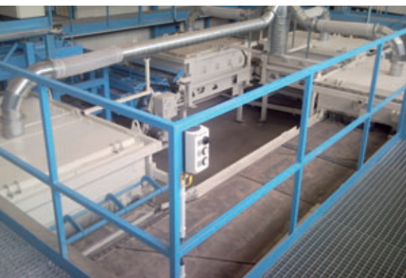
Overview of the Tumble Master with its 4 tumbling stations and block-layer turning device
