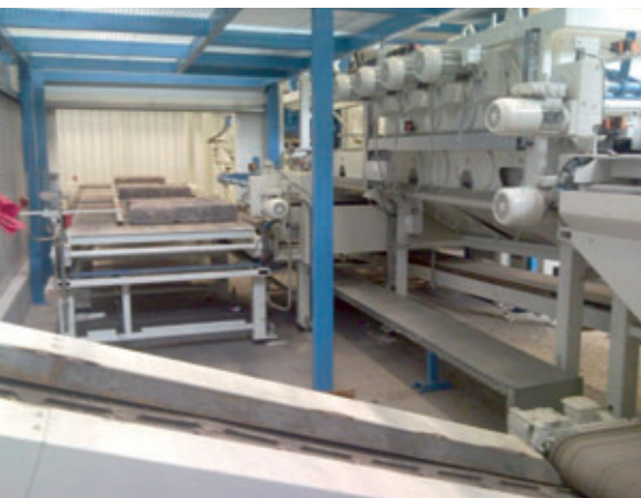
Circulating waste belts dispose of residual pieces
