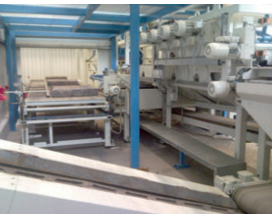
Circulating waste belts dispose of residual pieces
