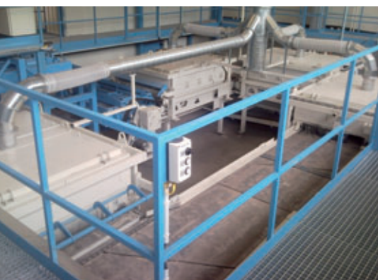
Overview of the Tumble Master with its 4 tumbling stations and block-layer turning device
