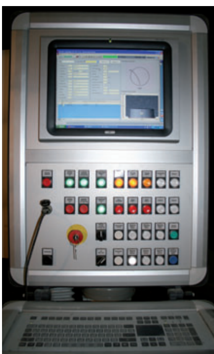
Control panel directly on the milling station
