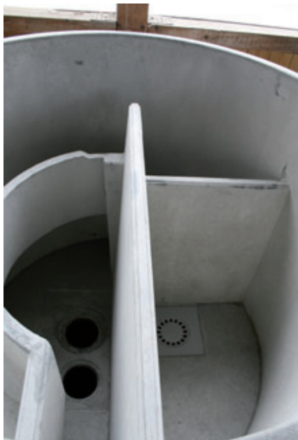
Inspection manholes for drinking water preparation have been part of the O. Wyss AG product range for many years
