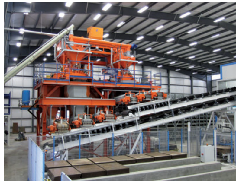
Fig. 6: The ACT MobilMat batch plant (in background) features a Twin Mixer Plant with a Wiggert HPGM 2250 and a HPGM 750 high shear mixer each feeding three concrete metering hoppers, allowing automatic mixing of three different colors for value added color-mix production of both color-thru and hard-faced paver products. The ACT MobilMat concrete batching system, equipped with the ACT HYDROMAT microwave water metering system for consistent water/cement ratio adherence, produces consistent and high quality concrete. The Hess system produces pavers and retaining walls on large steel production boards.
