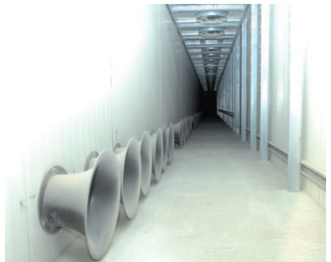
Ventilation system for large compartment
