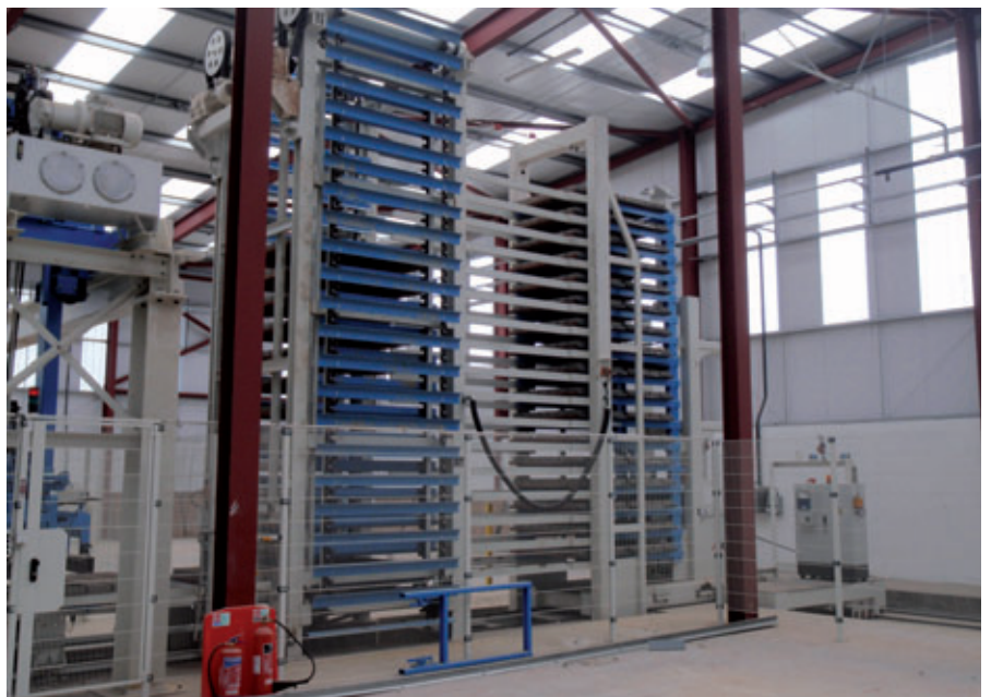
Dry side of the plant
