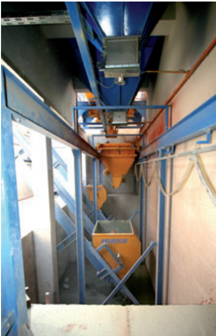
Masa Charging Scale and mixer bucket
