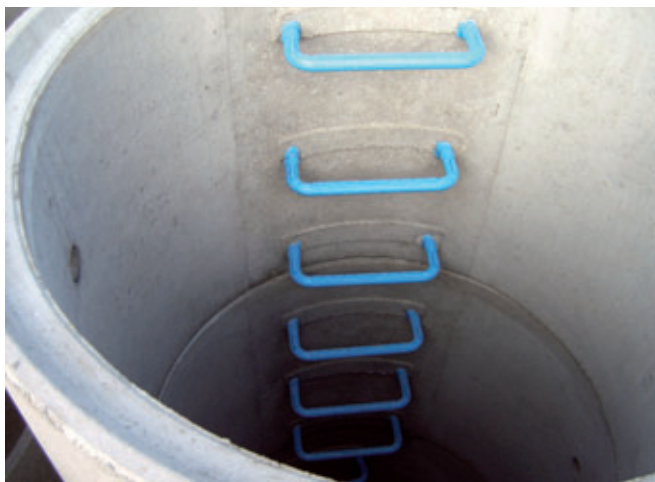
Manhole rings with manhole steps
