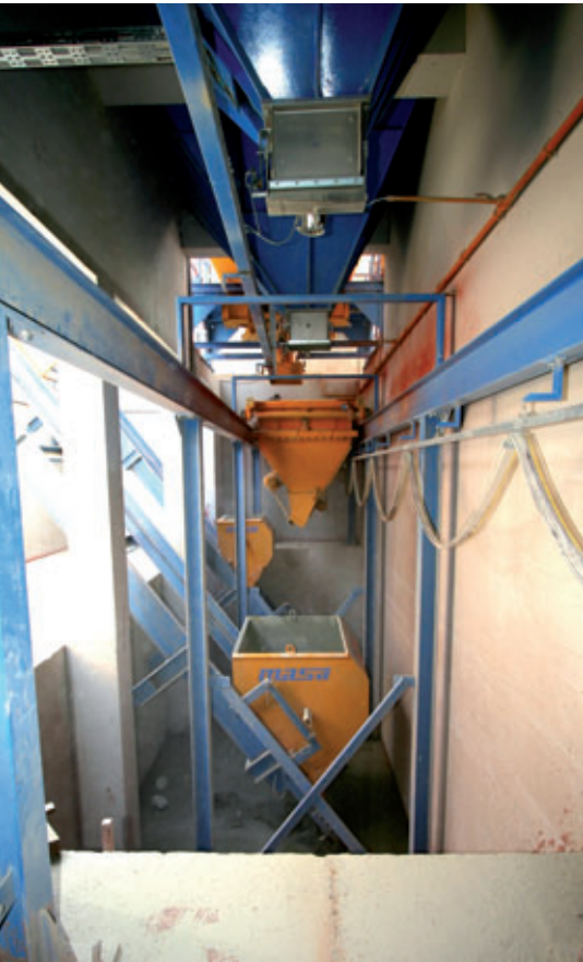
Masa Charging Scale and mixer bucket
