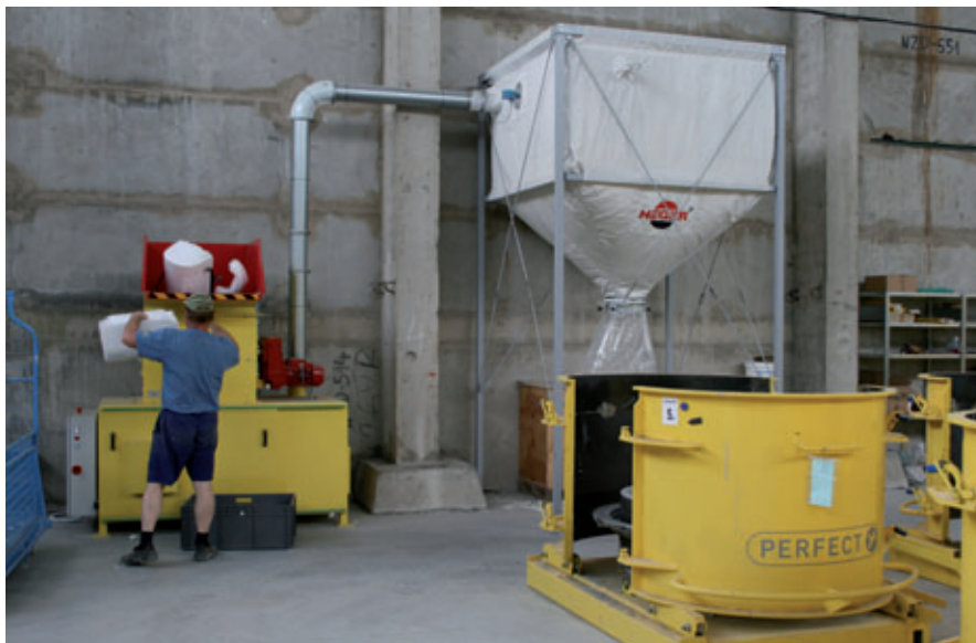
The removed EPS pieces are crushed in a shredding machine from Heger GmbH
