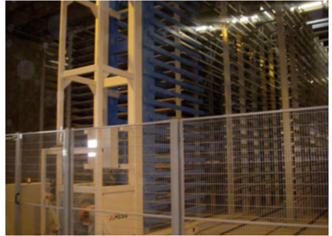
Hess finger car in front of the Rhotho rack system with a capacity of 5700 production boards
